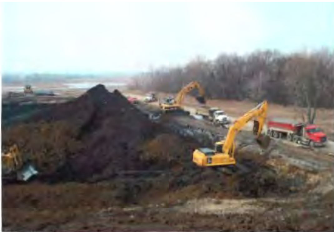
Loading out trucks and cleaning the side wall on the western portion of the ash pile
