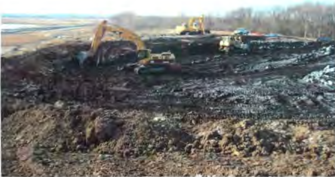
Excavating and moving ash from the southeast corner towards load out position
